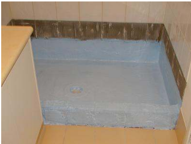
Leaking shower that has had the floor tiles and two rows of wall tiles removed. A Leak control flange has been fitted to the drain and the floor and wall have had Flexible waterproofing membrane applied.
