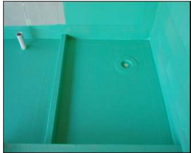
New shower recess where a Leak control flange has been fitted to the floor waste pipe and the floor & wall junctions reinforced with reinforcing bandage and finished off with Flexible waterproofing membrane.
