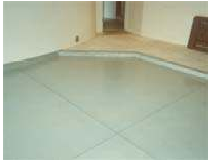
Balcony has had Flexible waterproof membrane applied & is now ready for tiling
