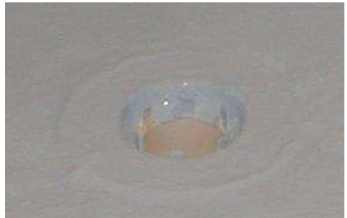
Leak control flange fitted to drain point
